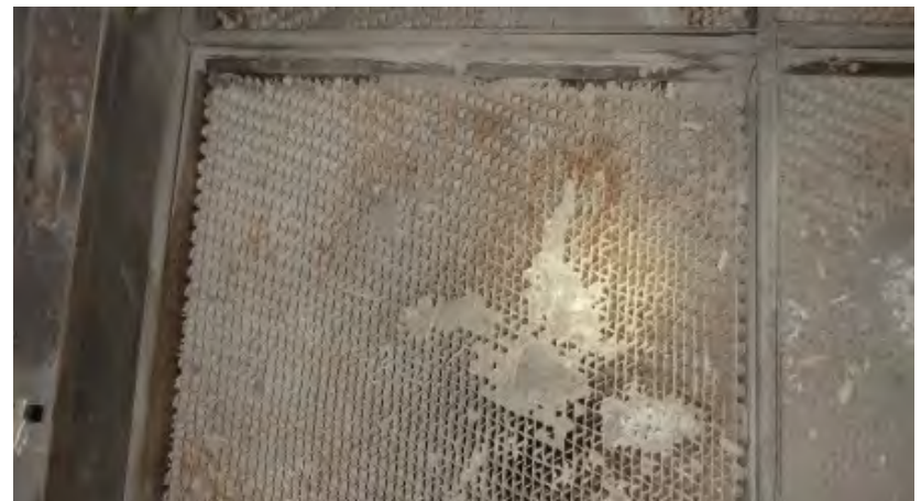
Corrugated Catalyst Pluggage Between Sub Layers & Inlet
