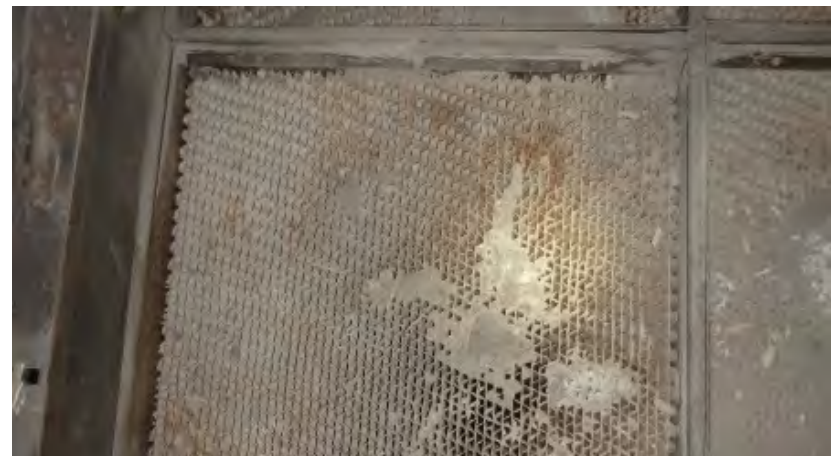
Corrugated Catalyst Pluggage Between Sub Layers & Inlet
