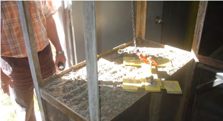
Plate Catalyst Pluggage Accumulates Between Sub Layers & Inlet
