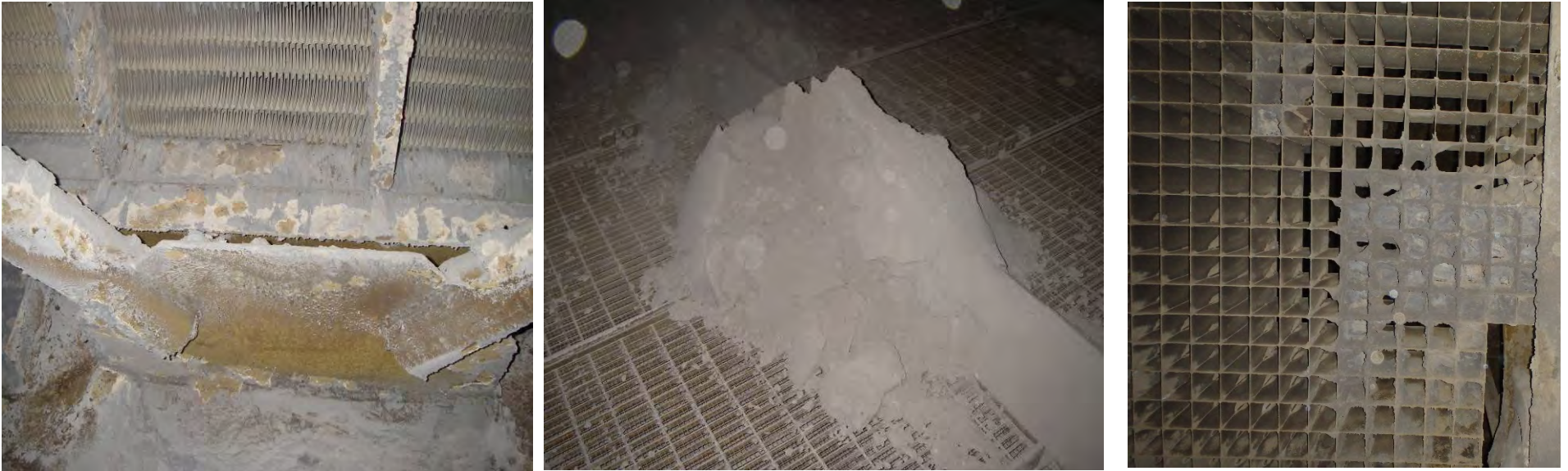
Fly ash pile located below gusset plate due to ash shear
