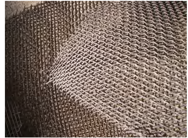
Coated & Non-Coated Screens Failed (High Velocity)
