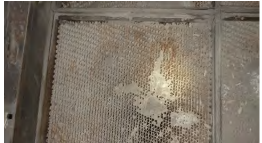
Corrugated Catalyst Pluggage Between Sub Layers & Inlet
